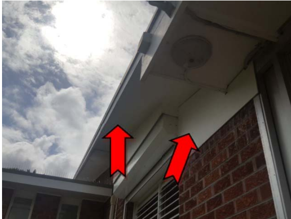
Photo 1. Exterior, throughout, eaves & fascia – suspected asbestos-containing fibre cement sheeting.
