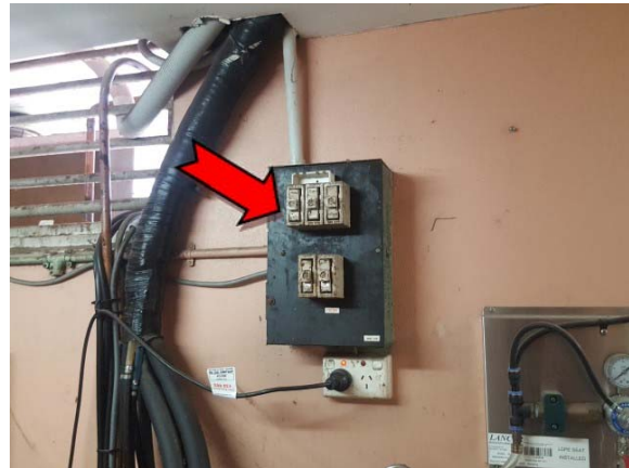
Photo 8. Interior, ground floor, rear storage area, electrical backing board – suspected asbestos-containing bituminous backing board.
