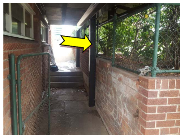
Photo 18. Exterior, throughout, features – suspected lead-containing green upper paint system.
