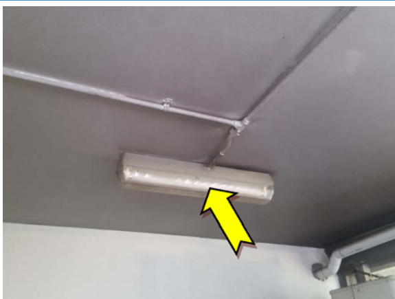
Photo 17. Interior, throughout, single tube fluorescent light fitting – suspected PCB-containing capacitor.
