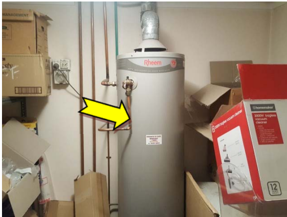
Photo 15. Interior, ground floor, east elevation, office, hot water heater – suspected SMF internal insulation.
