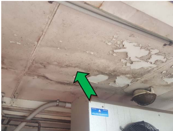
Photo 3. Exterior, north-west elevation, bin area, throughout, ceiling – non asbestos-containing fibre cement sheeting.
