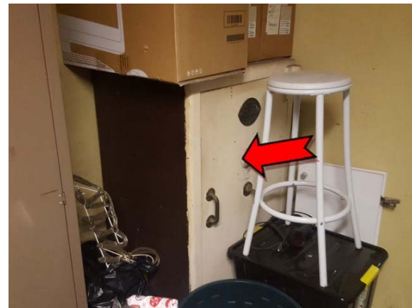
Photo 10. Interior, ground floor, rear storage area, safe – suspected asbestos-containing insulation material.
