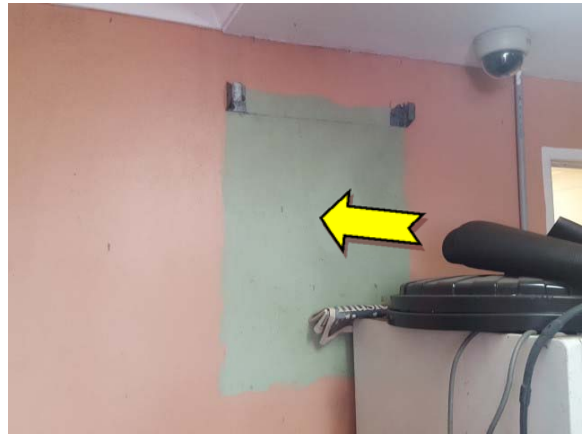
Photo 22. Interior, throughout, walls – suspected lead-containing lower green paint system.
