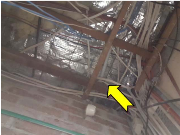
Photo 13. Interior, level one, throughout – suspected SMF sarking insulation.
