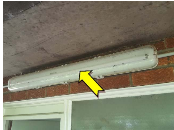
Photo 16. Exterior, throughout, single tube fluorescent light fitting – suspected PCB-containing capacitor.
