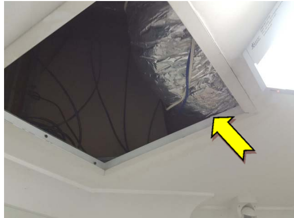
Photo 14. Interior, level one, throughout, flexible ductwork – suspected SMF internal insulation.
