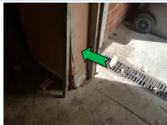
Photo 12. Interior, ground floor, doorway to exterior bin area, infill panels – non asbestos-containing fibre cement sheeting.
