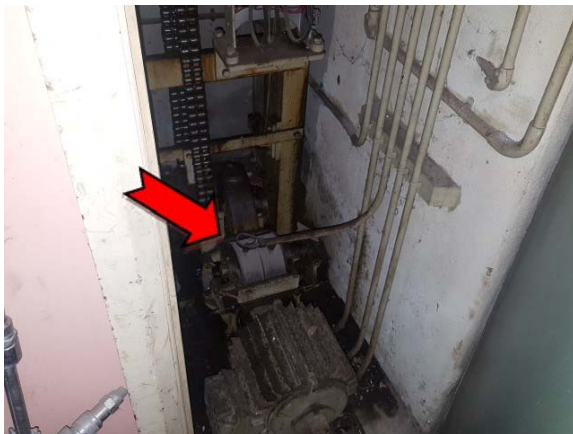
Photo 9. Interior, ground floor, lift motor – suspected asbestos-containing friction pads.
