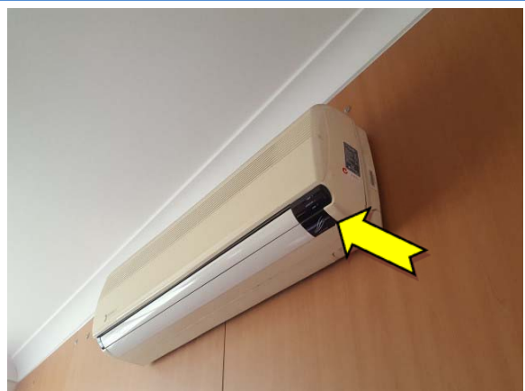
Photo 24. Interior, level 1, office, air conditioning unit, unknown refrigerant – suspected ozone depleting substance.
