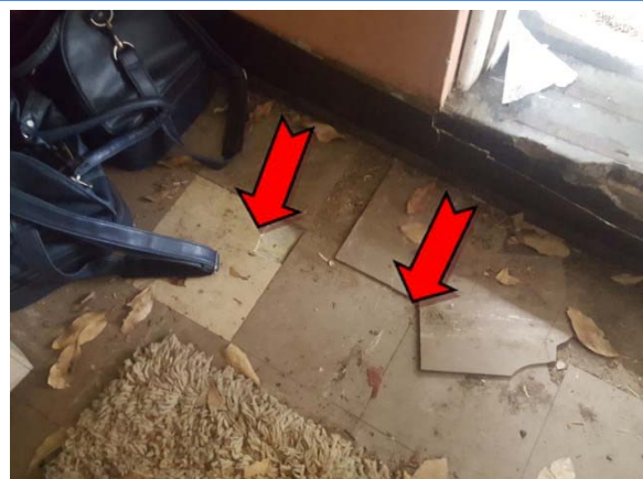
Photo 6. Interior, ground floor, bowls storage room, beige and white floor coverings – asbestos-containing vinyl floor tiles.
