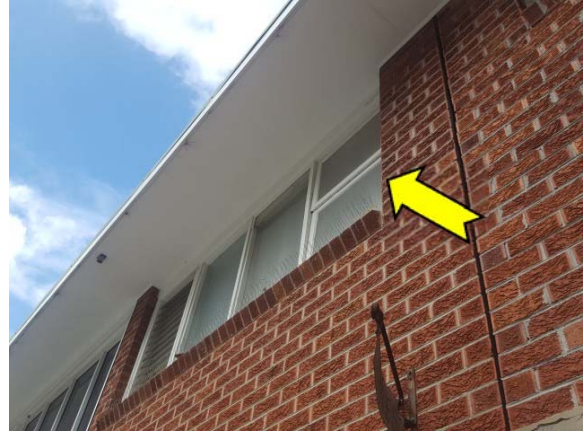
Photo 20. Exterior, throughout, eaves and window frames – suspected lead-containing white upper paint system.
