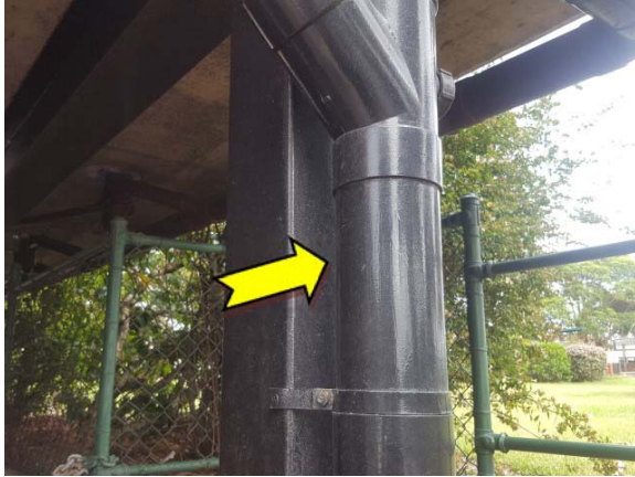
Photo 19. Exterior, throughout, features – suspected lead-containing black upper paint system.
